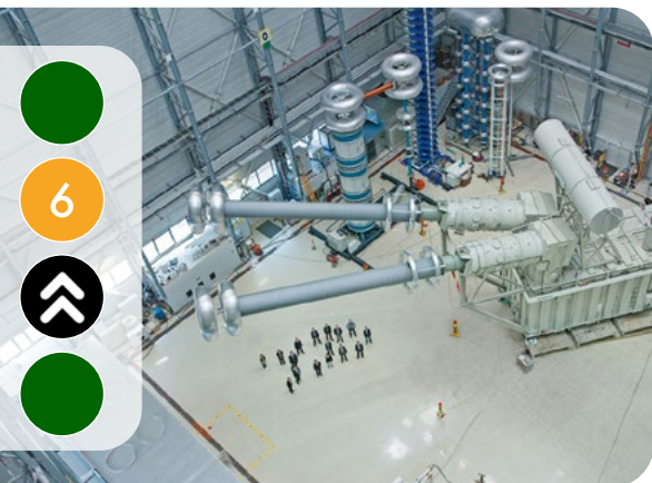
World's first 1,100 kV HVDC transformer, Siemens
